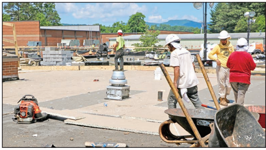
Workers getting the new roof on the main building of the Towns County middle and high school. Photo by Mark Smith
